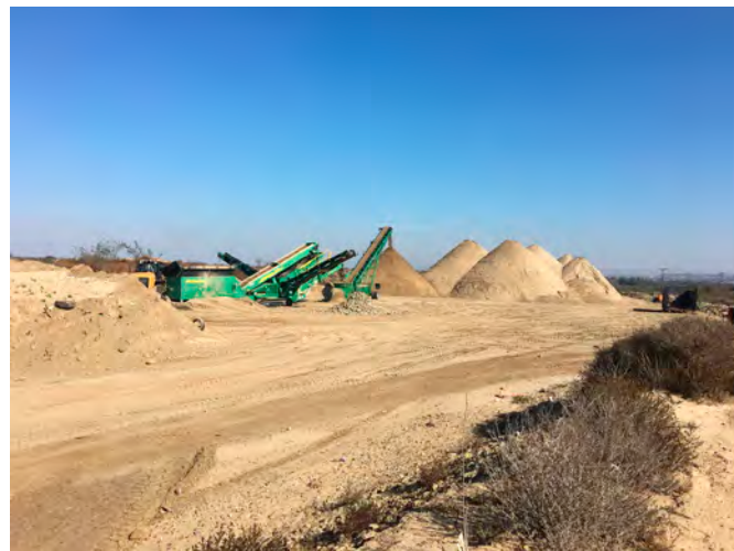
Cleared and processed sediment from the basin being prepared for transport off site.
