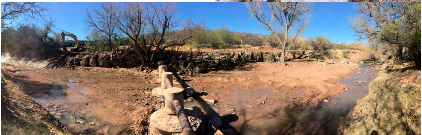
Before and after cleanup photos in the Santa Cruz River in Nogales, Arizona.
